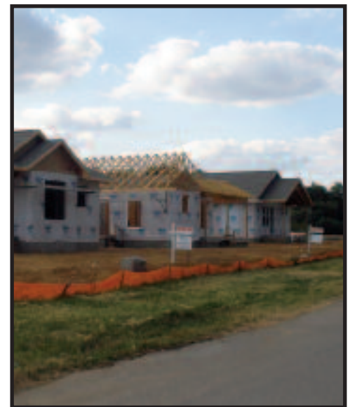
Homes started going up in Shadewood Place in June and are expected to be completed sometime next year. When finished, there will be 19 Habitat homes and up to four market-rate homes built by Bussing Construction.
