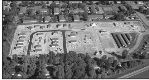
The infrastructure construction on the New Haven Subdivision began in 2007 along with 27 houses.
