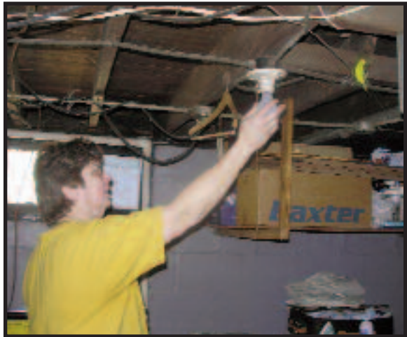
Volunteers from Vectren, Crossroads Christian Church and the Glenwood neighborhood began weatherizing homes on Feb. 15. Volunteers helped homeowners install energy efficient light bulbs in all the homes.
